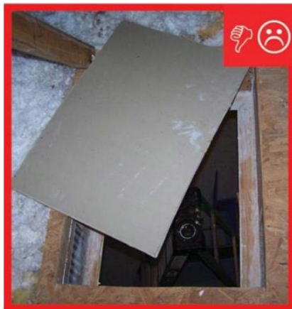
Attic access panel is not insulated or gasketed
