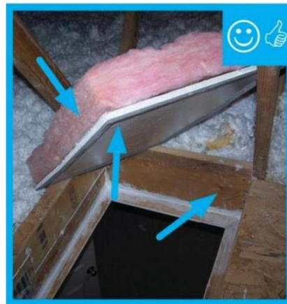
Access panel is insulated and gasketed; this is acceptable as long as insulation is mechanically fastened to cover
